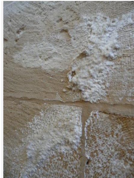
Efflorescence de surface
